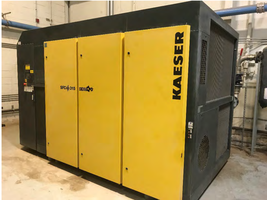
Kaeser Air Compressor
