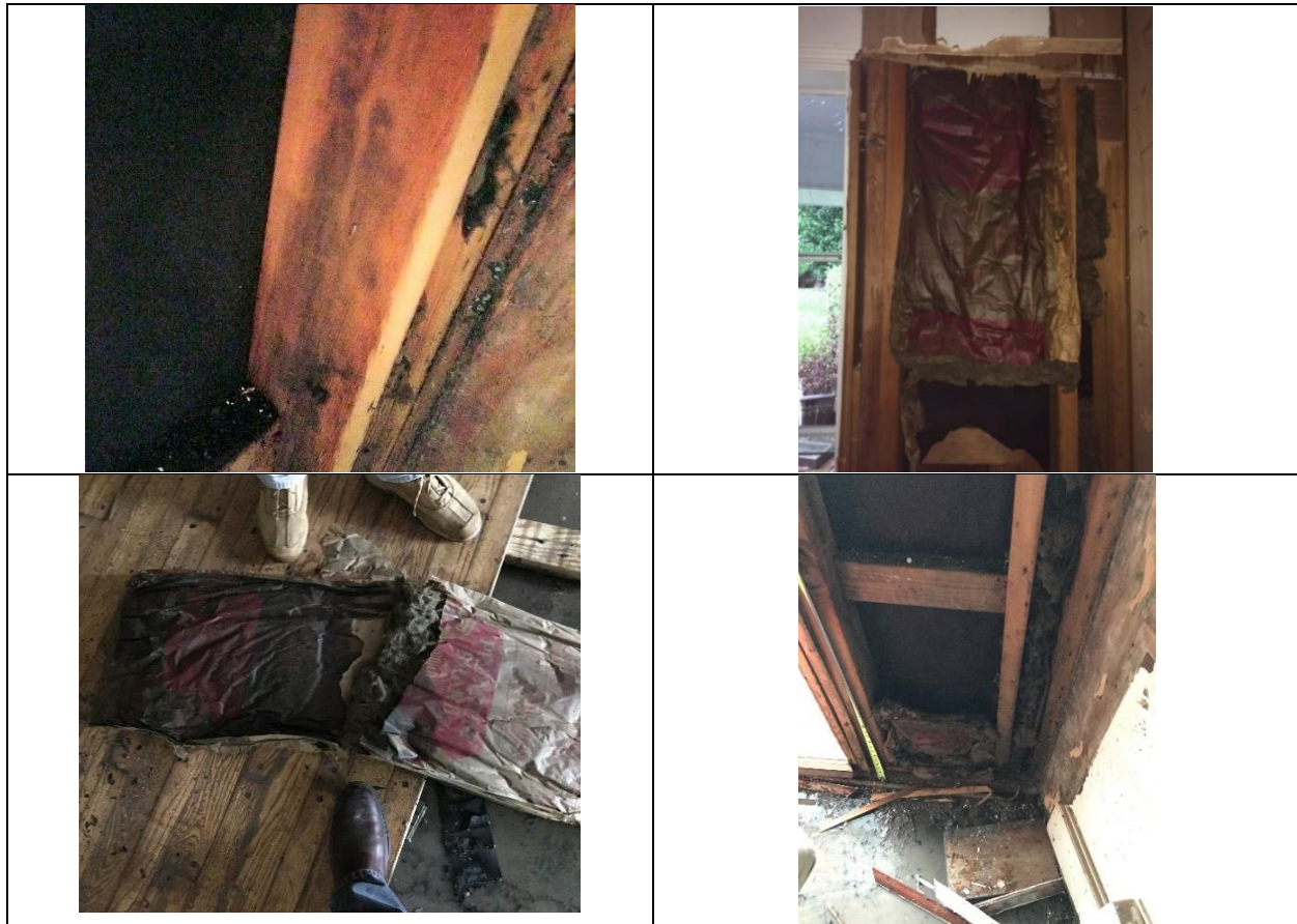
Note transition from wet to dry indicating lack of wicking
