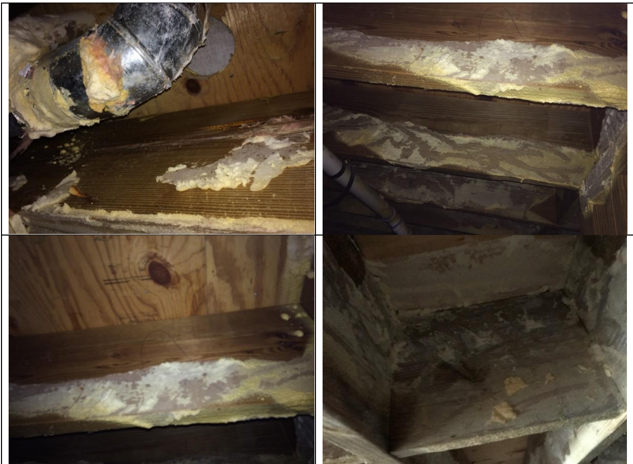
Note how OC SPF appears to have been applied from above leaving air gap between top of foam and bottom of subfloor sheathing in pictures
